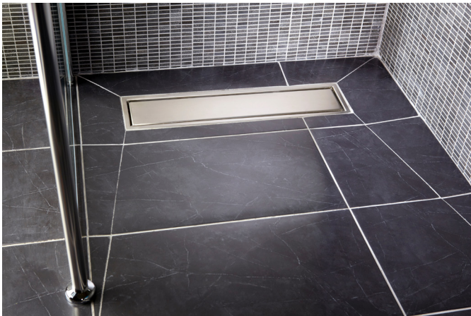
Linear drain—cover showing.
