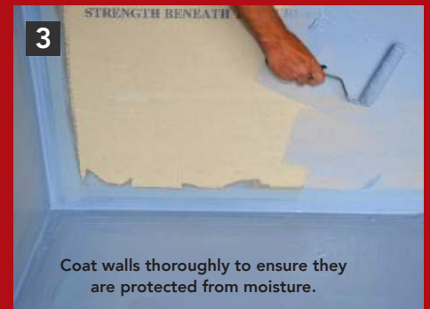
"Tank" the shower base and walls with two full coats of waterproofing.
